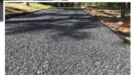
Spread fill material level to the top of the PRO PLUS cells.
