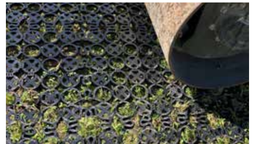
Use compacting equipment – heavy rolling compactor, plate compactor, jumping jack, and hand tamper – to press ROOT into the soil.
